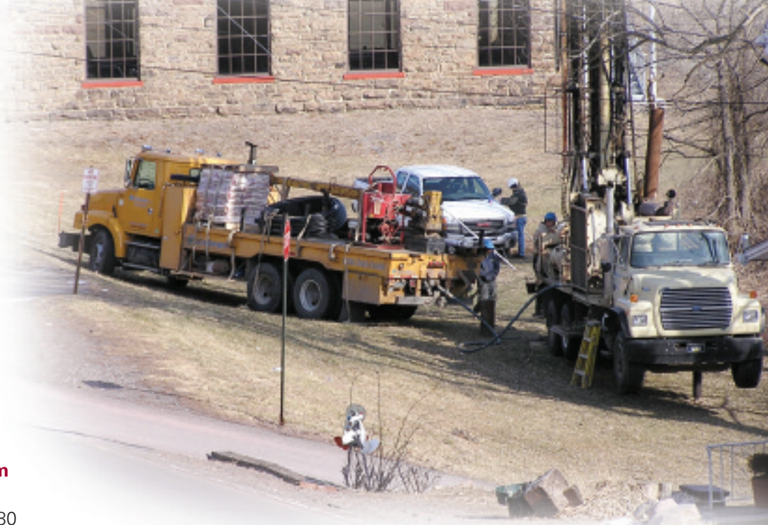
A large drilling rig was used to develop the test site for the new geothermal system to be installed in 2011.
